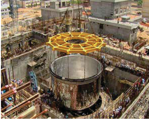
Prototype Fast Breeder Reactor (PFBR) at Kalpakkam, India
